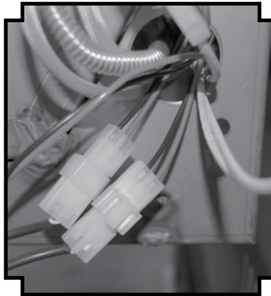
Figure 7-1 - Transformer connection point on left rear grill frame.
