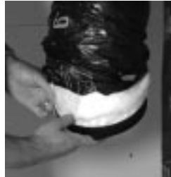
figure 10.3 Insert insulation inside the collar and finish by taping the vapor barrier on the collar.
