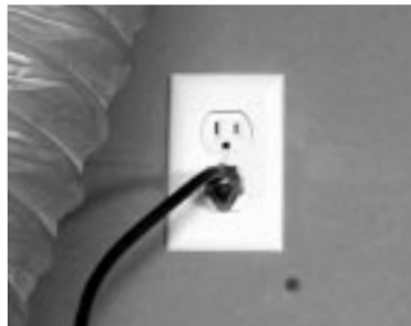
figure 9.2 Electric Wall Outlet
