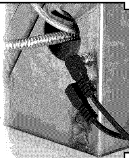
Figure 7-1 - Transformer connection point on left rear grill frame.
