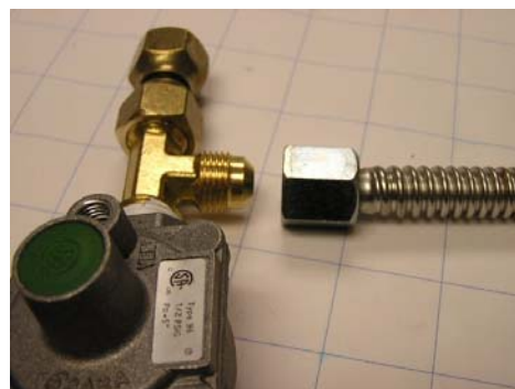
Natural Gas Connection between Flex Connector and Regulator Assembly
