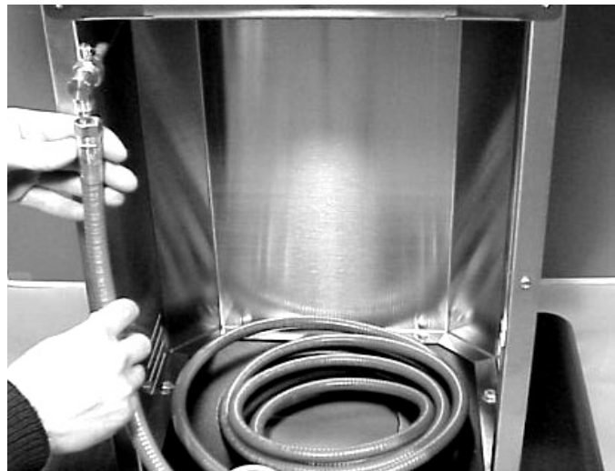
Figure 16 Natural Gas Hose Connection
