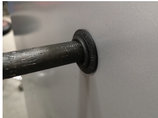
FIGURE 27 - FURNACE GAS PIPE CONNECTIONS (NOTE RUBBER GROMMET)
