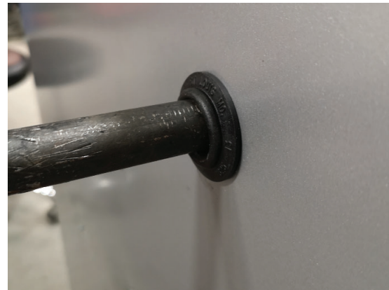
FIGURE 27 - FURNACE GAS PIPE CONNECTIONS (NOTE RUBBER GROMMET)
