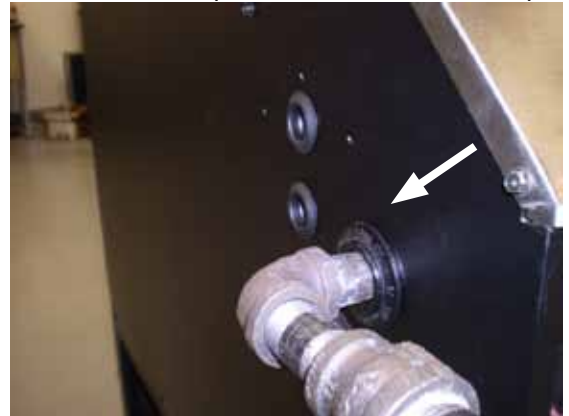
FIGURE 28 - FURNACE GAS PIPE CONNECTIONS (NOTE RUBBER GROMMET)
