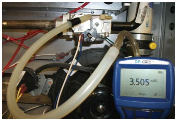
FIGURE 30 - MANOMETER MEASURING GAS MANIFOLD PRESSURE
