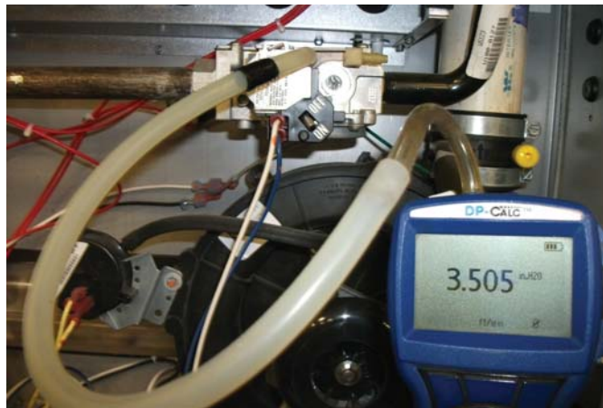
FIGURE 30 - MANOMETER MEASURING GAS MANIFOLD PRESSURE
