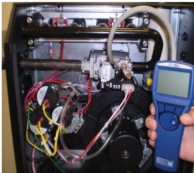
FIGURE 30 - MANOMETER MEASURING GAS MANIFOLD PRESSURE
