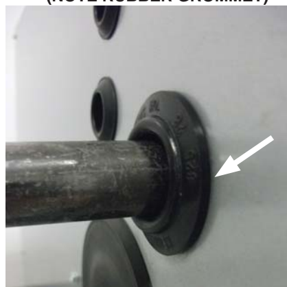
FIGURE 27 - FURNACE GAS PIPE CONNECTIONS (NOTE RUBBER GROMMET)
