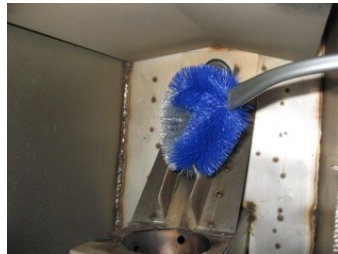
Figure 2: Pellet Slide Cleaning
